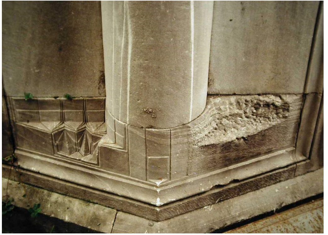
Unfinished muqarnas workmanship in the corner of Mehmed III Mausoleum. Photo by Gülsün Tanyeli.
